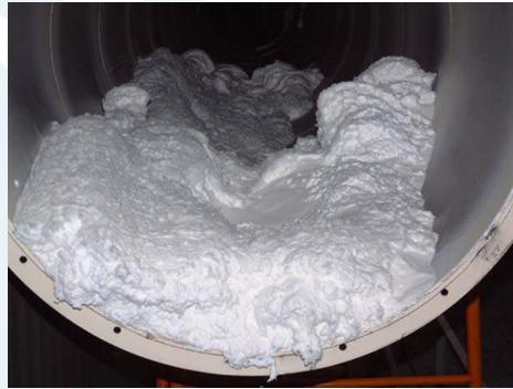
Figure 18 Material Accumulation Inside a Duct Due to Low Air Velocity
